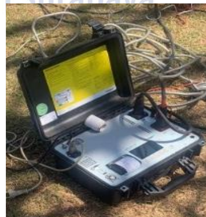
Gambar 4. Alat Leakage Current Monitoring (Sumber: Gardu Induk 150 KV Kenjeran Surabaya, 2022)
