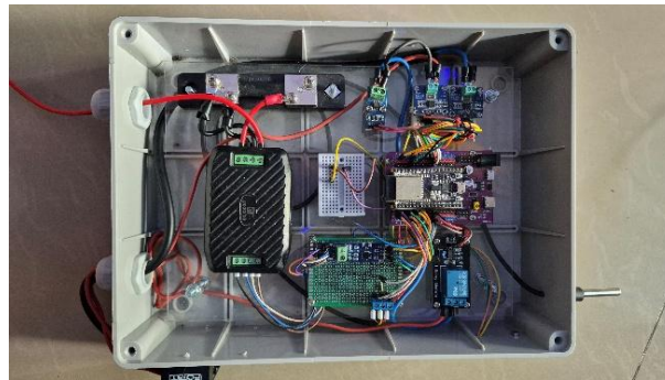
Gambar 5 Box Kontrol Monitoring
